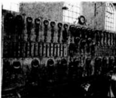
MAIN SWITCHBOARD, RILAND ROAD 1910.
