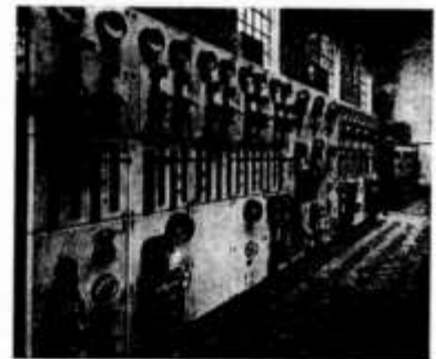
MAIN SWITCHBOARD, RILAND ROAD 1935.
